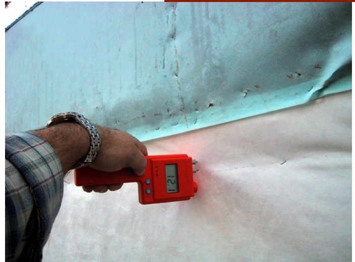
High vapor permeable housewrap with low moisture reading on OSB under the DuPont™ Tyvek® HomeWrap®
